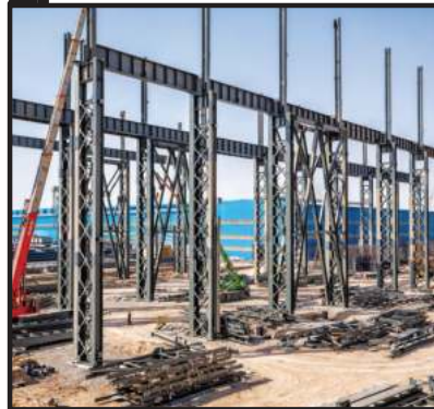
Steel framework of the smelting plant of the Sepid Farab Kavir Steel Complex
