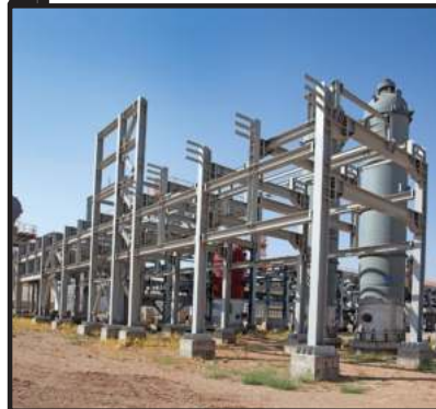
Steel structures of ammonia plant of Kermanshah Petrochemical Industries
